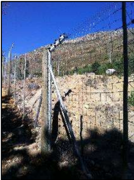
Figure 18: A sand mound along the Zwaanswyk Fence which baboons used to gain access over the fence.
